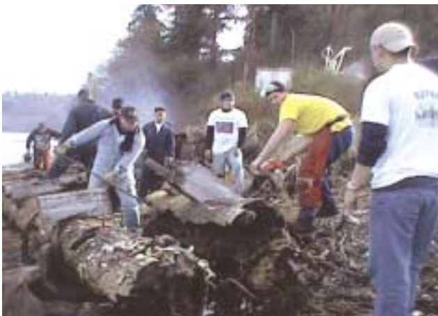
Shoreline cleanup project: Crew from the USS Camden dismantling old dock near Bangor, Washington.
